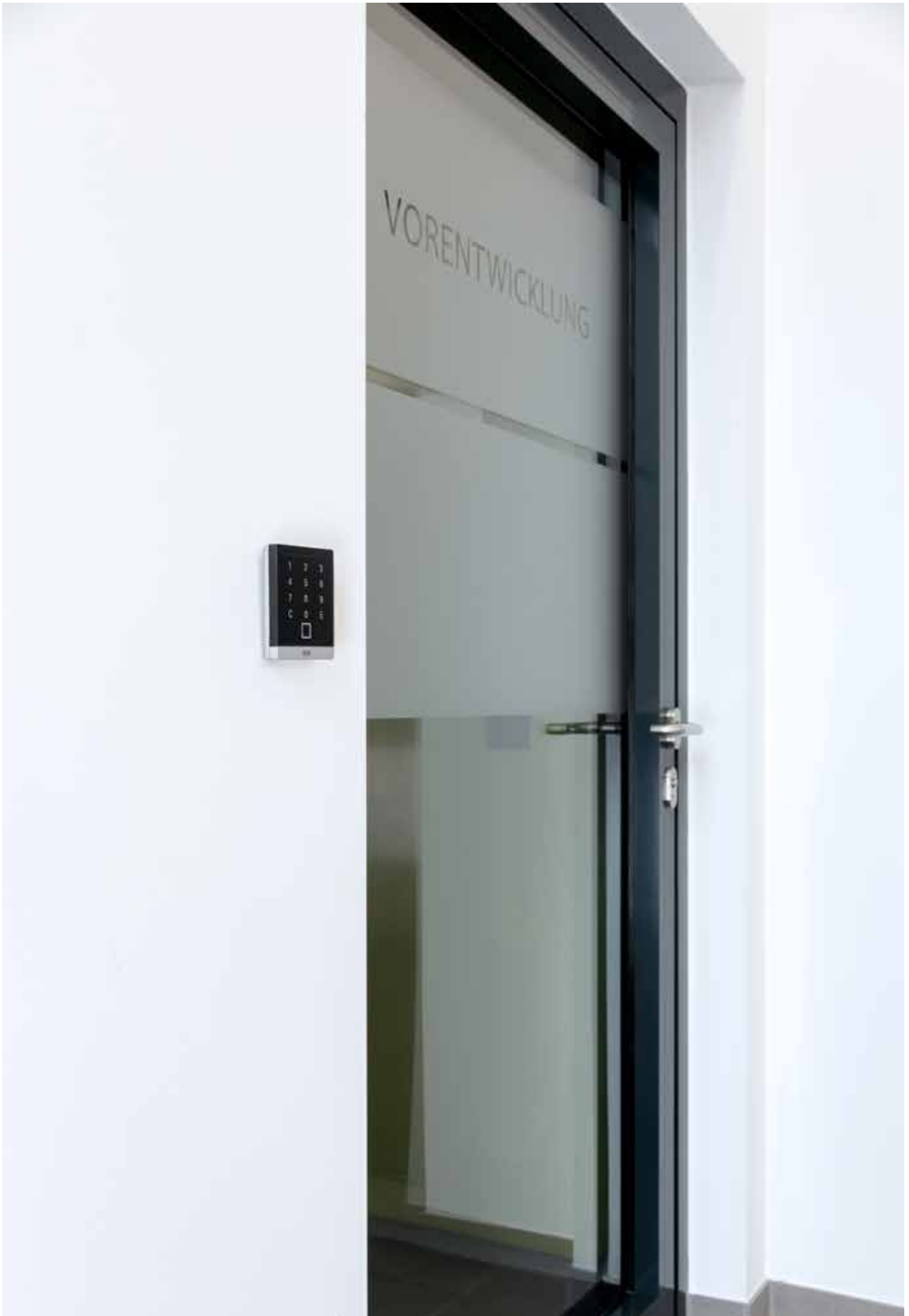
Installation situation, GCVR 800 Touch T, Germany (photo: GEZE GmbH)
